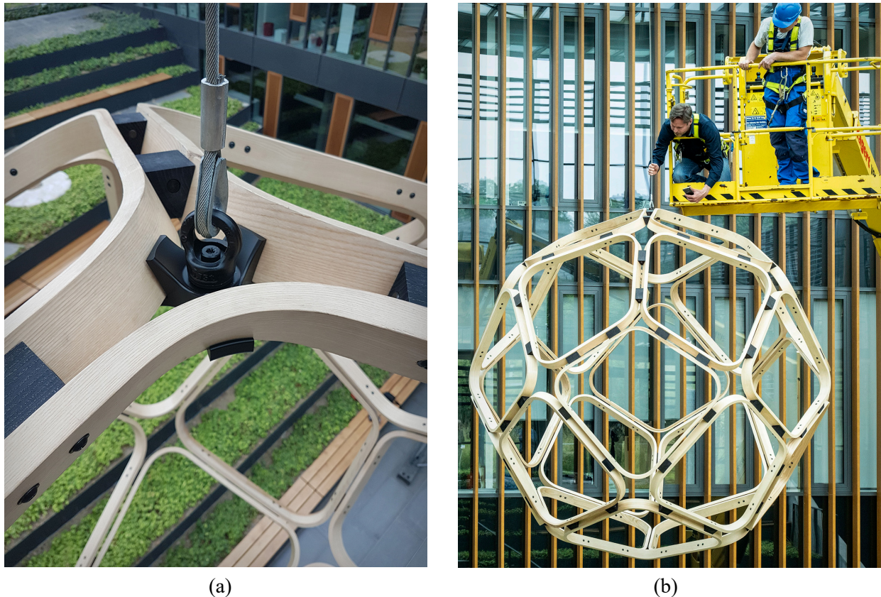
Figure 3: Installation of BenDit: (a) Hook, (b) Cable check. Photographers: DL (a), Sven Geise (b).
