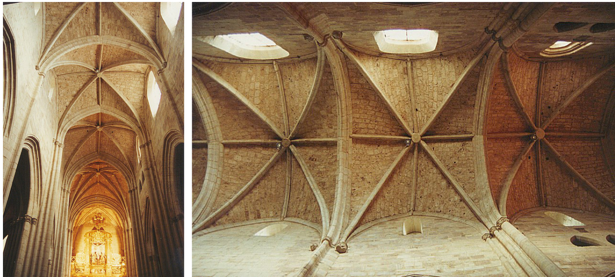
Figure 1: Main nave of the Church of Santa Maria la Real, Najera, Spain. A geometric analysis of the church shows the vaulting system to be completely distorted. Arches and vaults are deformed, the walls and columns are bent and cracks appear in the aisles. Geometry is the first test to verify the structural state of a Gothic construction.
